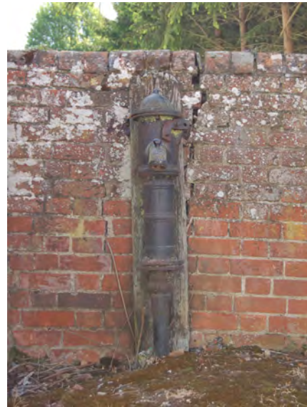
Picture 1.19 Any opportunity to repair the village pump would be beneficial.
